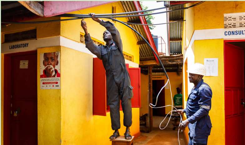
Cables are installed throughout the clinic creating a secure network.
